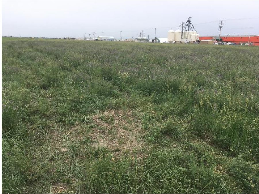
Photograph 6 – Bore Hole on West Side of the Property Facing Southwest Note the bore hole was installed days before for a geotechnical investigation related to developing the Property.
